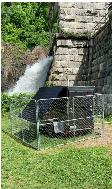
Example solar powered SATT system within a locked temporary fence.
